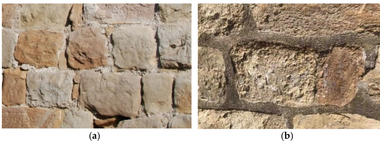
Figure 1. Malpractice of introducing cement-lime mortar in Serbia (a) before July 2012; (b) nine years after repair of the wall—July 2021).
