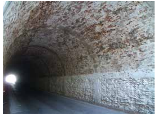
Figure 11. Gorgoracha Tunnel, Granada (1848). Author: Antonio Jiménez Torrecillas, 2005. Source: Antonio Jiménez Torrecillas Studio.
