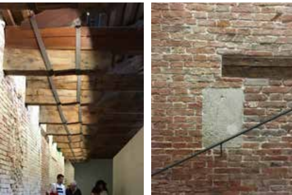
Figure 11. Restoration of the wooden trusses and evidence of cuci-scuci techniques. Credit: Photos by Francesco Bianchi
