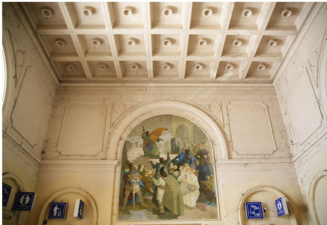
Fig. 191 / Giurgiu railway station in a neglected state (Author: C. Vărzaru)
