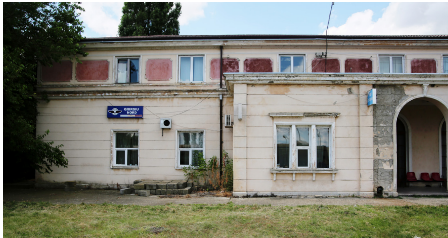
Fig. 227 / North railway station in Giurgiu – abandoned heritage (Author: C. Vărzaru)
