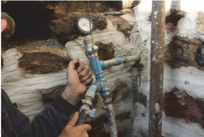
Figure 3. Injecting the injection mixture into a wall, using a nuzzle consisting of a manometer and a three-way valve that is used for returning unused mortar injection into a tank – mortar injection recirculation
