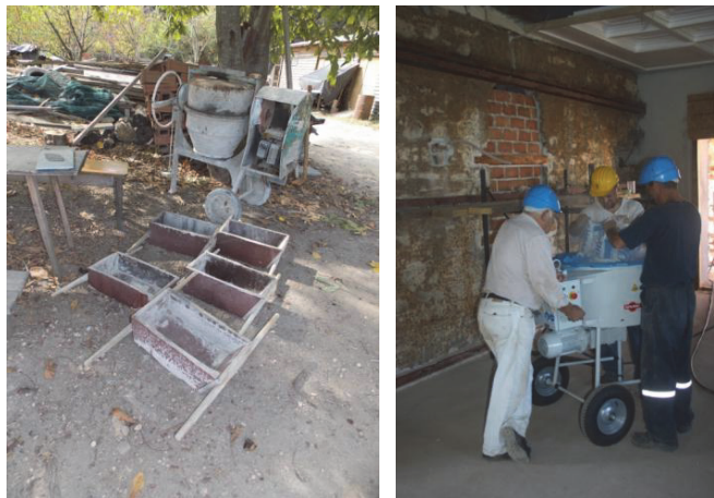
Figure 1. Mortar mixers for making injection mortar: a) standard rotating drum mixer and volumetric measure for determining the ratio of material, b) planetary mortar mixer without a rotating drum
