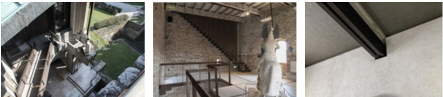
Figure 9: Application of contrasting materials to the refurbishment of the castle in Verona (Castelvecchio).
