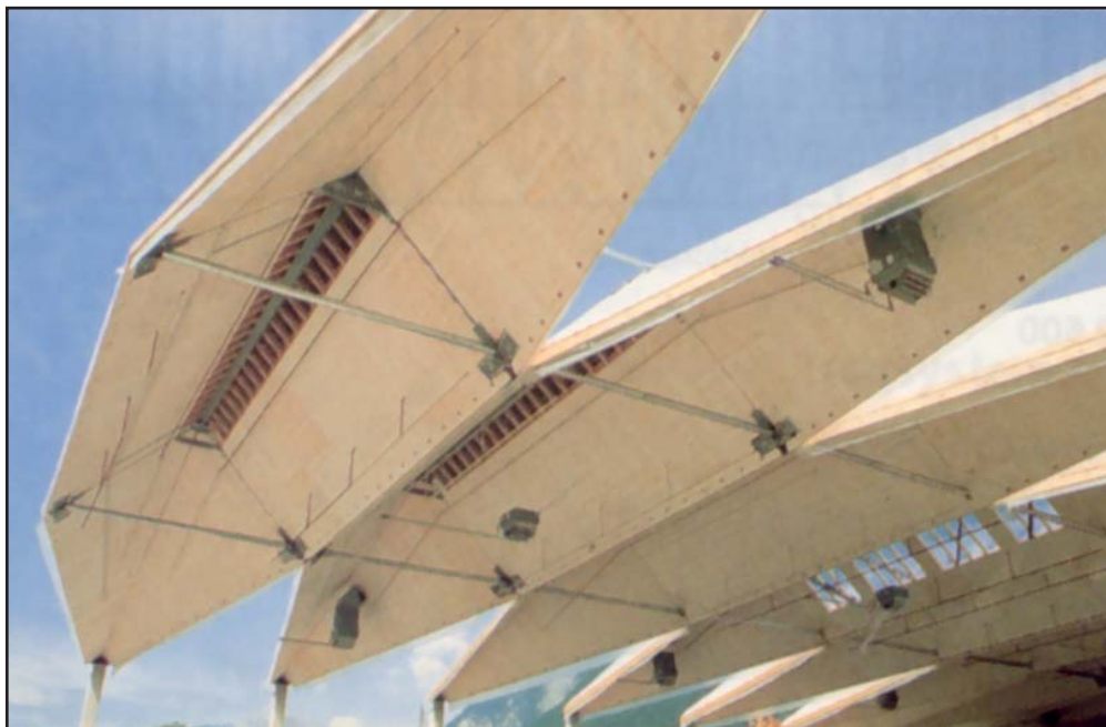
Figure 1. The roof of the factory hall constructed as a wooden panel folded construction, span 43.60 m, the architect Josef Lackner, Jenbach, Tyrol, Austria, 1996.
