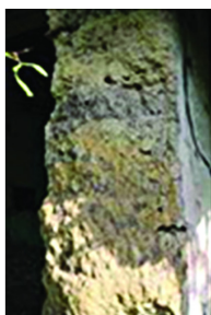
Figure 3. Cross-section of the rammed earth wall with clearly defined different layers of rammed earth; abandoned house in Perlez
