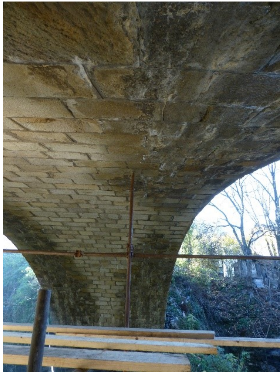
Figure 6. Elevation of the arch barrel where deterioration of alternately built-in stone blocks and the visible difference between the central-dry and side-wet sides of the arch barrel.
