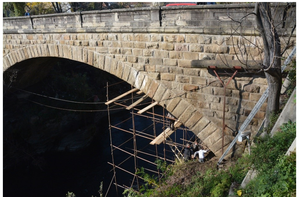
Figure 5. Elevation of the spandrel and wing wall with arch ring showing the dimensions and relation between stone blocks from which it was built and their current state.
