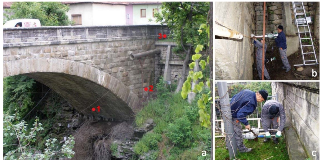
Figure 11. Taking a drilling sample for laboratory analysis: (a) positions of samples, (b) process of sampling the wing wall and (c) process of sampling the stone fence.
