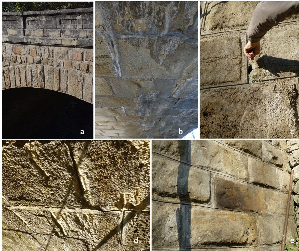
Figure 12. Close-up of bridge structure: (a) decolorisation of the parapet and spandrel wall, (b) forming of white stains and edges, (c) sampling for biological analysis, (d) efflorescence of arch barrel and (e) change of colour on the wing wall.
