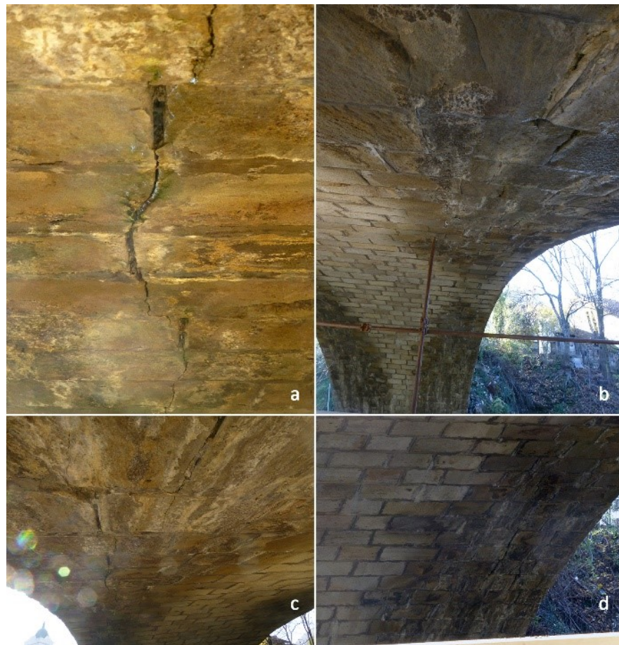
Figure 7. Photos of arch barrel cracks (a) between and through stone blocks, (b) on the wet side of the arch barrel, (c) through binder and (d) on the lower third of the arch barrel.
