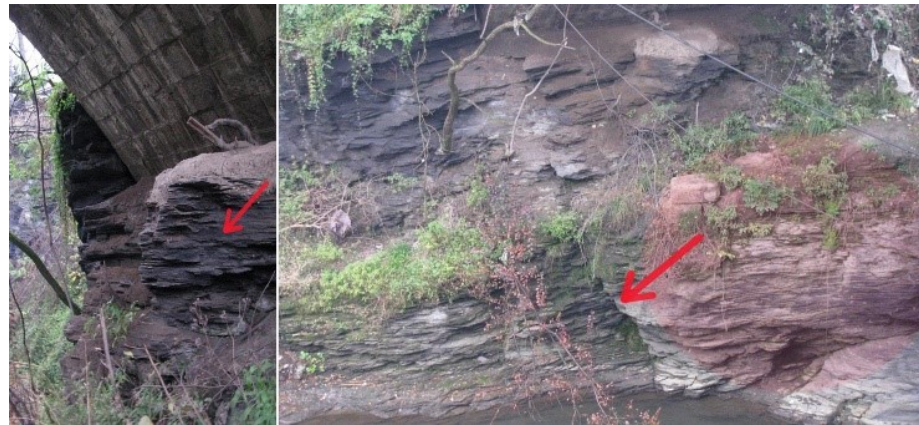
Figure 8. Cracks and rift in the rocky mass under the bridge foundation observed at site.
