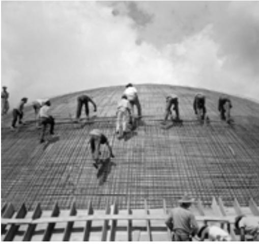
Figures 2-3: National Congress, Brasília, The Construction of Brasilia, photos by Marcel Gautherot.
