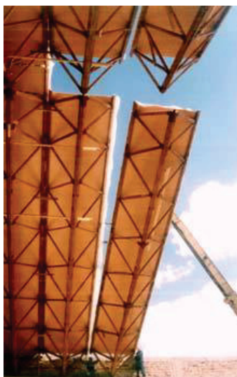
Fig. 10. Installation of packages of folded bearers, Sports Hall in Medveđa, the designer of the construction LKV Center, 2001. [27]
