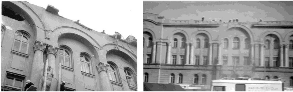
Figure 2. Significant constructive devastations appeared after earthquake of 1969. [10]
