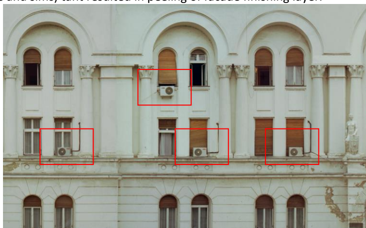
Figure 3. Condition of the main facade before restoration process. [9]
