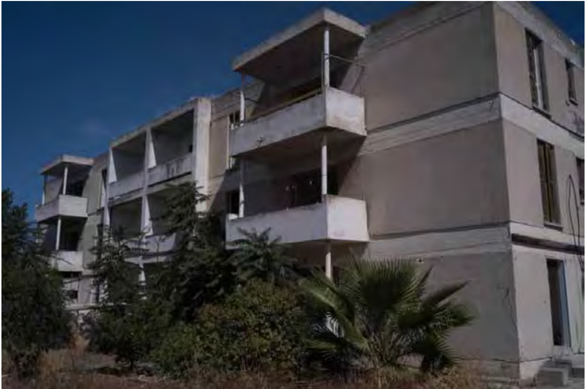
Figure 3. Typical deterioration of building stock as it exists today.
