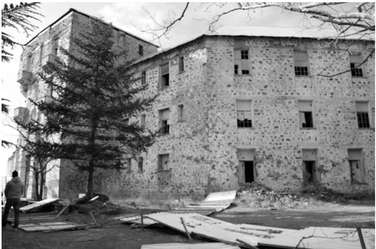
Figure 2. The abandoned façade of the Berengaria Hotel, 2011. Source: U-SHer Project ©
