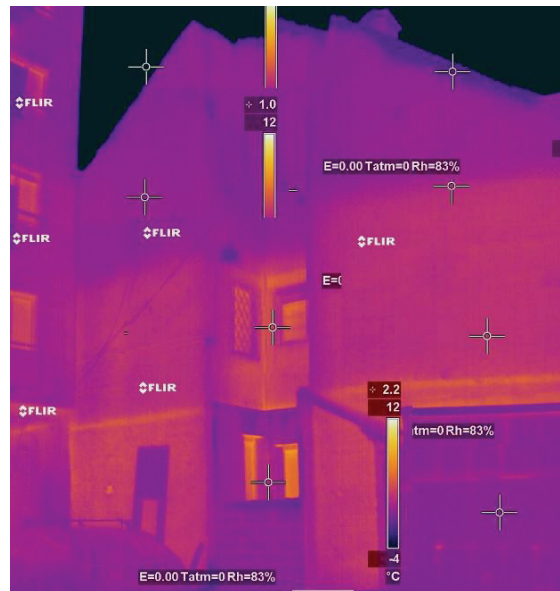
Fig. 3 Thermovision image of side (gable) wall
