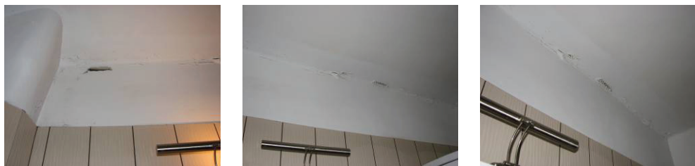
Fig. 4. Photo bathroom interior (junction: wall – ceiling)
