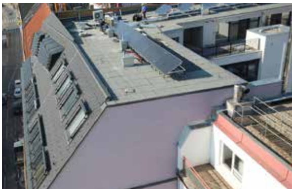
Figure 2. A solar thermal system located on the roof of the building.
