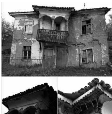
Figure 5. The house of Mile Cenkov, 1912, village of Smilovci (the entrance façade and the details of the holker eaves, below, credits: G. Ljubenov)
