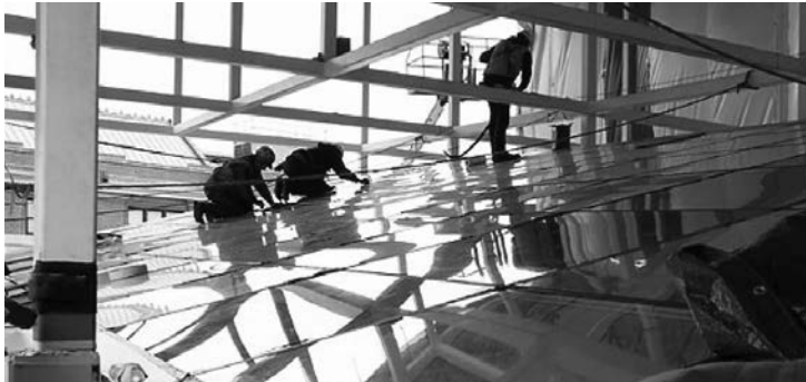
Figure 1 The glass curtain wall of the Wexner Center was overhauled to restore light to galleries darkened by an earlier quick fix.
