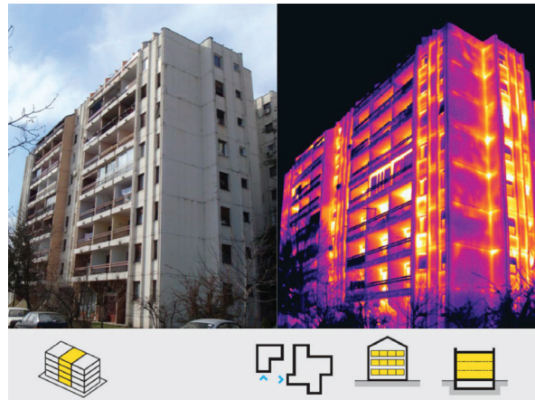
Figure 4: Building_02; conventional (top left) and infrared image (top right); National Typology type F4, characteristics shown below
