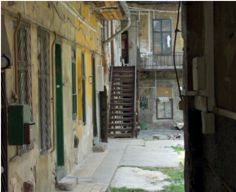
Figure 2: Typical inner courtyard in the Corvin area before the planning intervention.
